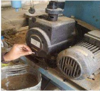
Figure 3 : Oil contamination within Purge Pump
