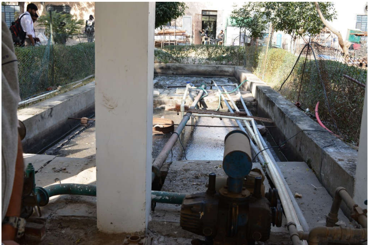
Fig: - Visit of Water Treatment Plant by Students at the Campus
