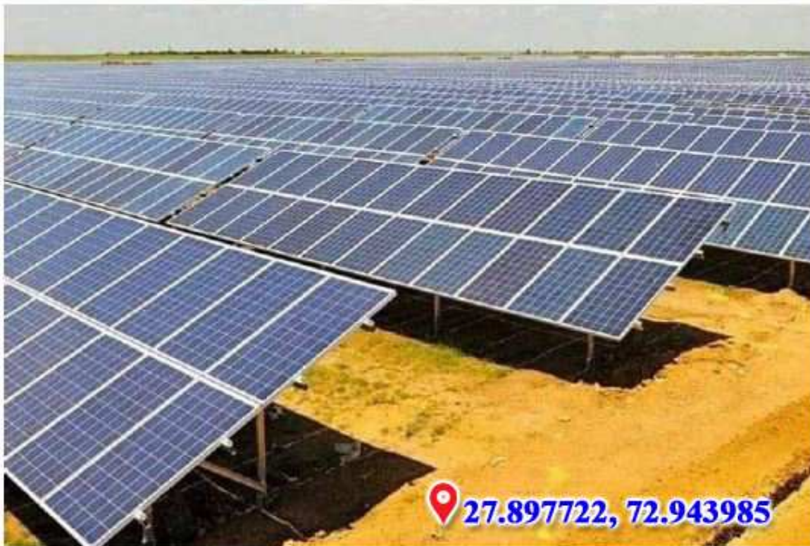
Captive Solar Power Plant at Kolayat
