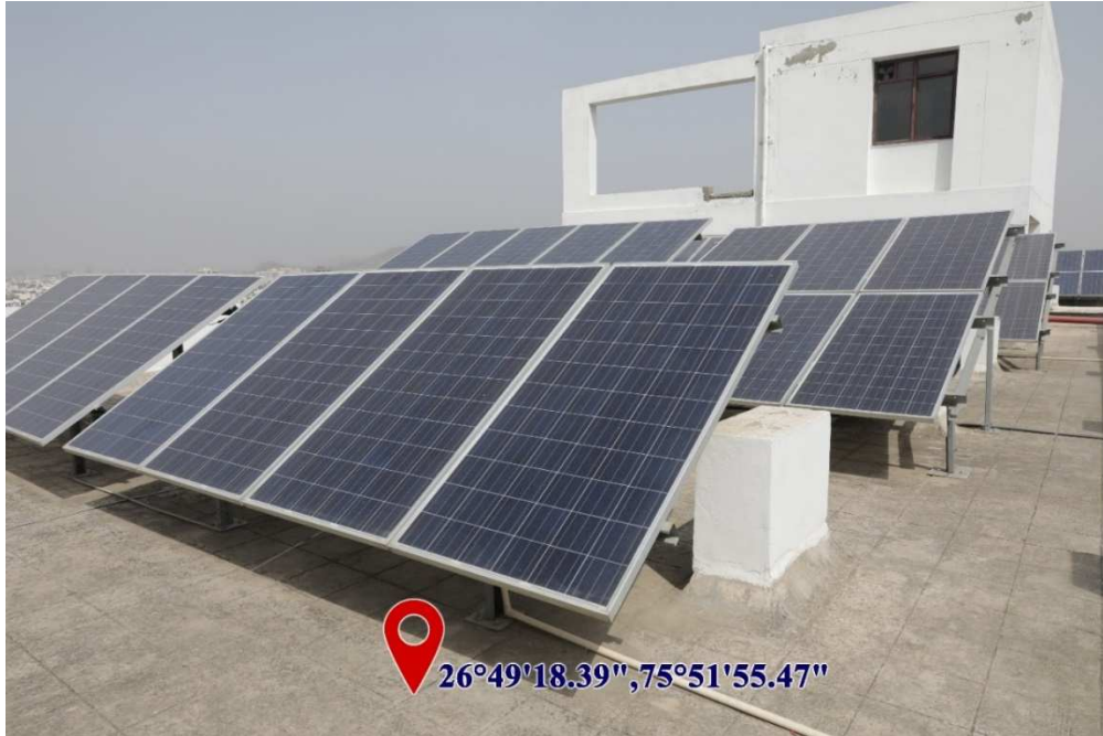
Geotagged Photograph of Solar Power Plant
