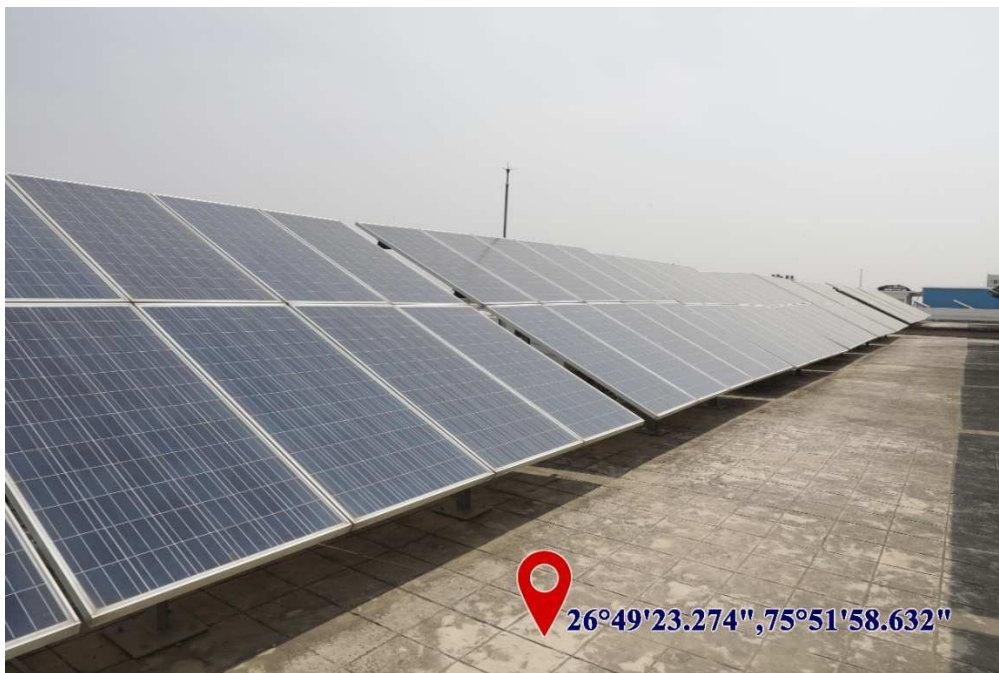
Geotagged Photograph of Solar Power Plant
