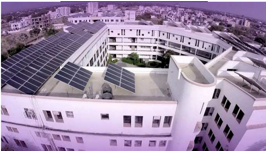
Photograph of Solar Power Plant
