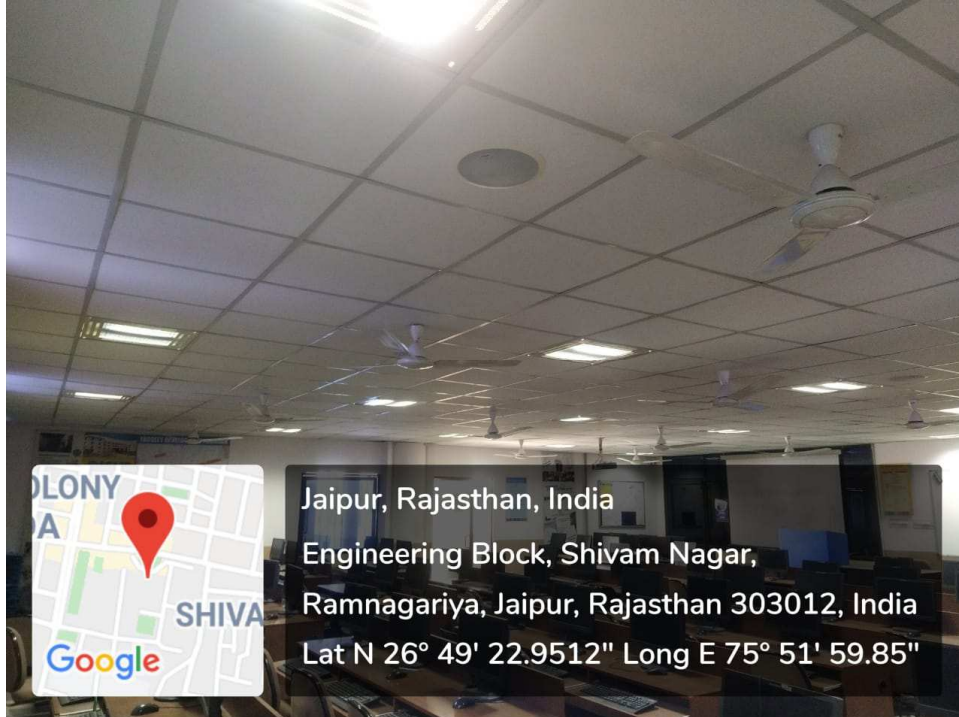
Use of LED Bulbs/Lights in Class Room & Labs
