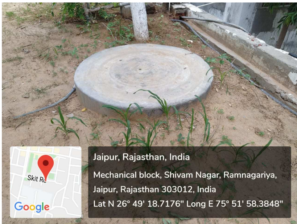
Liquid Waste Management System (Septic Tank)
