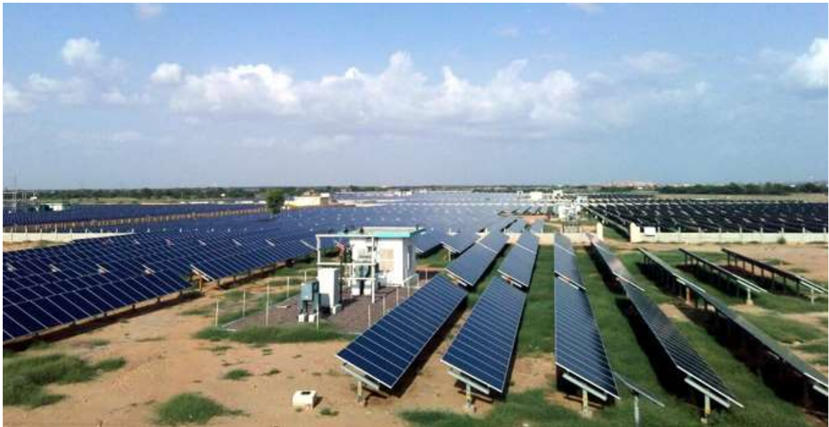
Photo- Solar Power Plant, Bikaner (500 kW Captive)
