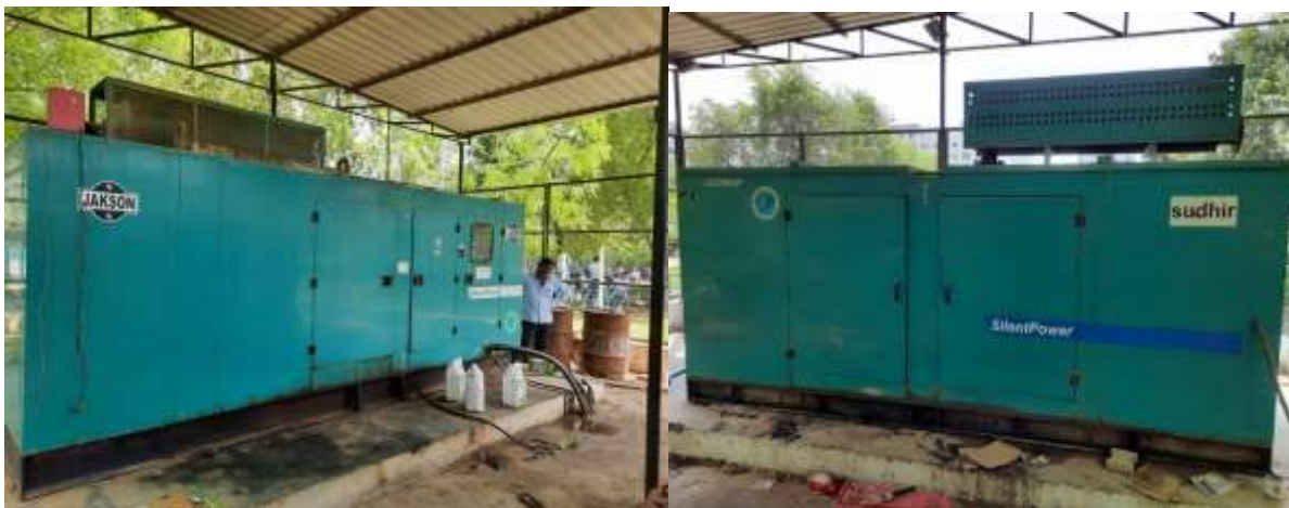
Photo- Diesel generators installed near Gate No.2
