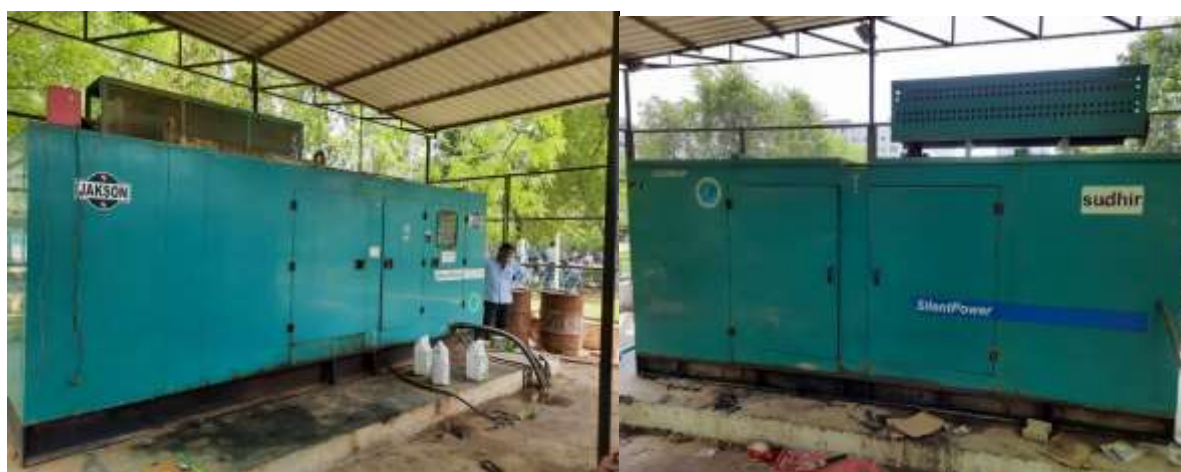
Photo- Diesel generators installed near Gate No.2
