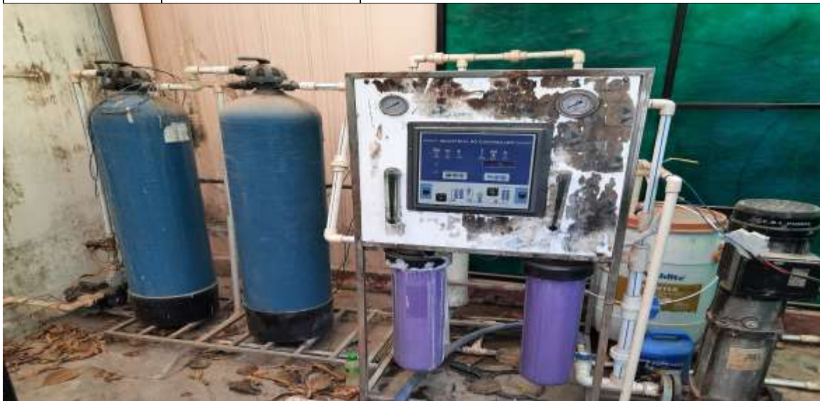
Photo-RO System in SKITM&G
