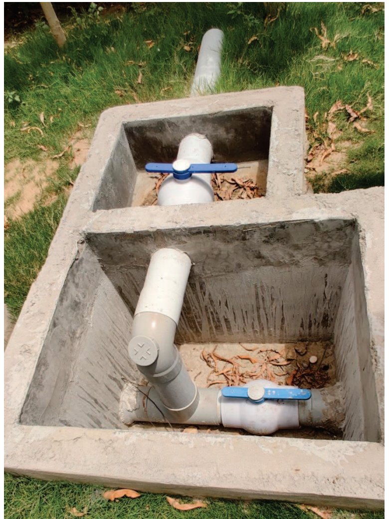
Rainwater collection system at SKIT
